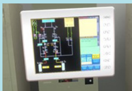
Virtual operation panel of gas cylinder cabinet
