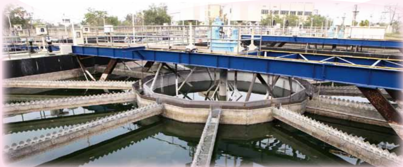
Construction Completion of Stage 2 of Phase 1 of the Waste Water Treatment Plant at the Kaohsiung Science Park (April 16, 2012)
