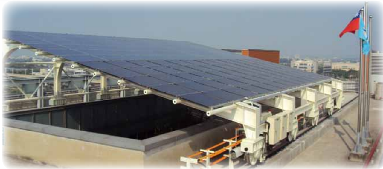
Energy Saving and Carbon Emission Reduced Photovoltaic Equipment on the Veranda of the STSP Administration Building at the Tainan Science Park (January 10, 2012)
