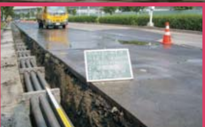
Completion of the 2008 Broadband Pipeline Installation Project at the Tainan Science Park
